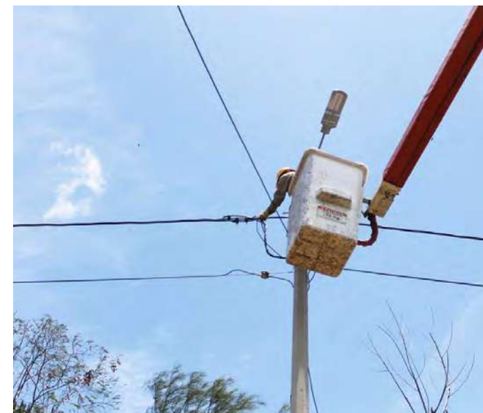
▲ Colombian LED Street Lighting Project
