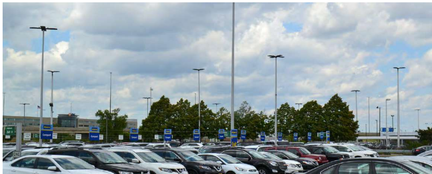
American Parking Lot LED Lighting Project ▲
