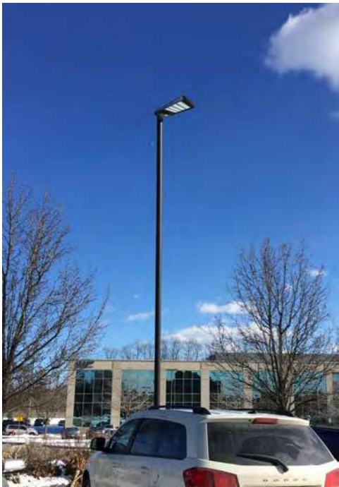
American LED Street Light Lighting Project ▼
